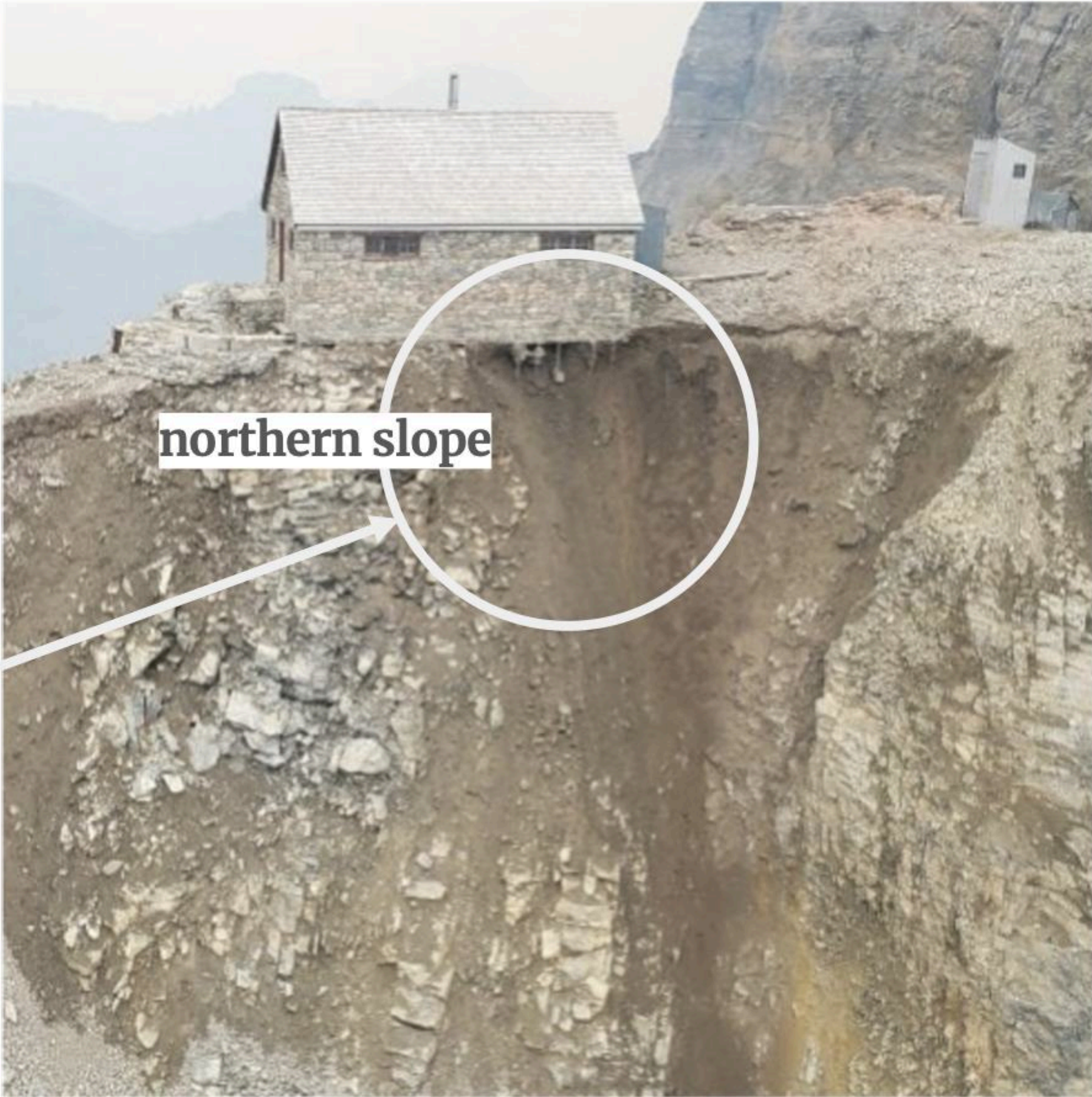
The Abbot Pass Hut and the erosion in 2021 . Photo: Parks Canada
